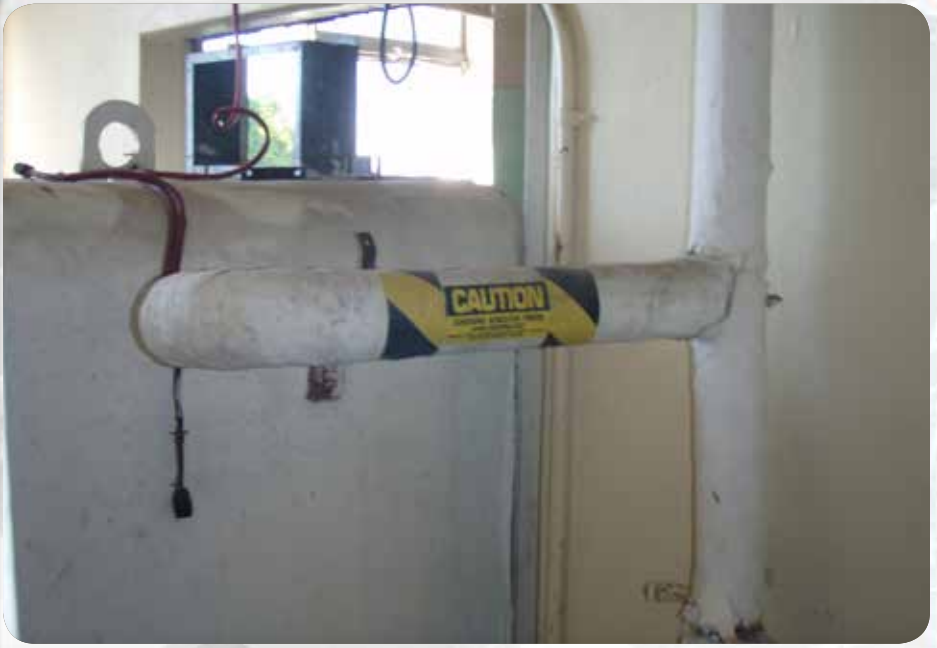
Lagging – for pipes or boilers
