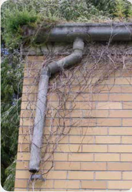
Guttering and down pipes
